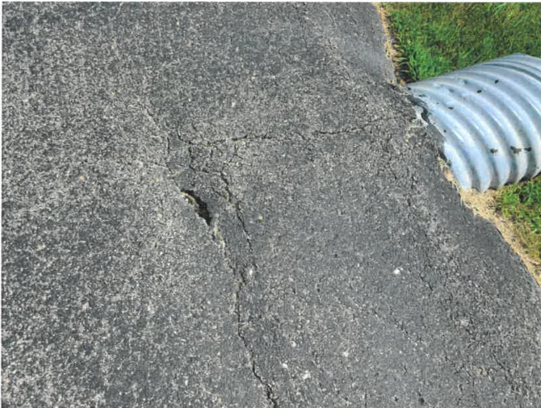
Close up of hole on east end of driveway apron.
