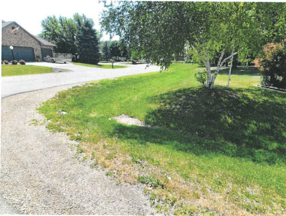
Looking south at the southwestern intersection of Royaltroun and Augusta. Just to the left of the dead spot in the grass is the roadside culvert.
