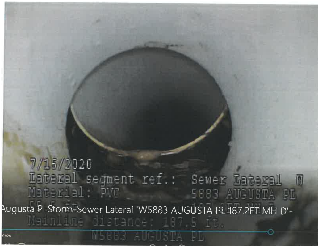
W5883 Augusta Place storm lateral. Lateral is active and connected but offset in the connection was noted at approximately 55-feet into the property from the mini storm.
