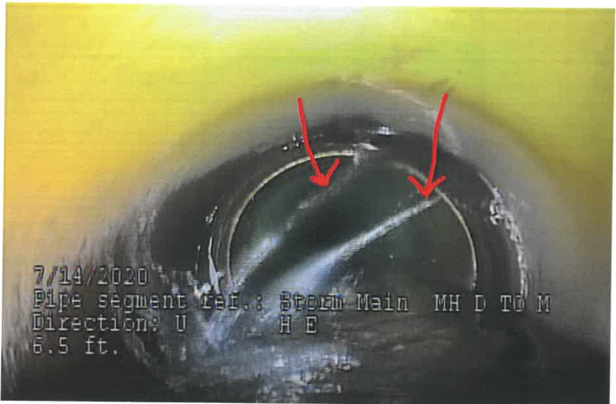
Infiltration visible near Manhole D at the corner of Muirfield and Augusta. The arrows point to the water infiltrating at the joint.
