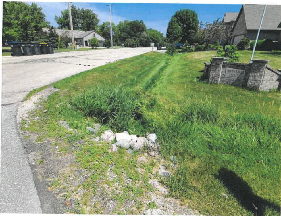
Looking north along the eastern ditch of Northshore Rd. There is a corrugated drain tile installed along this section of ditch that appears to be draining a sump discharge.
