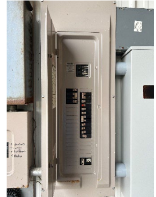
Main Electrical Service
