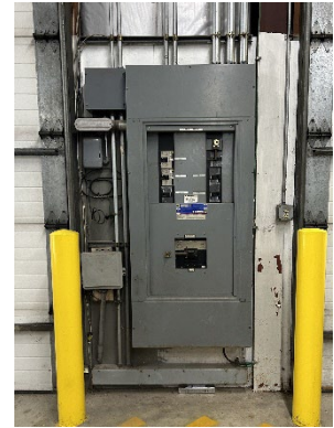
Main Electrical Service
