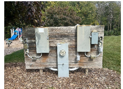
Additional Electrical Service
