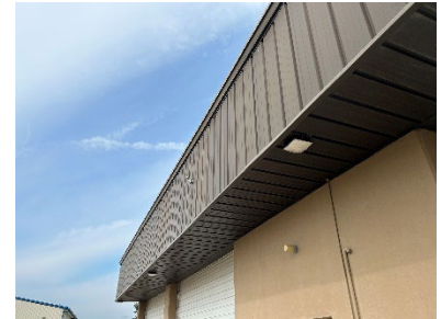
Existing LED Fixture & Photocell
