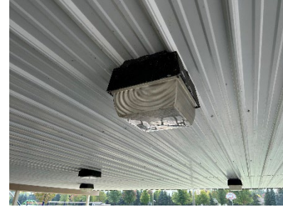
Existing HPS Lighting
