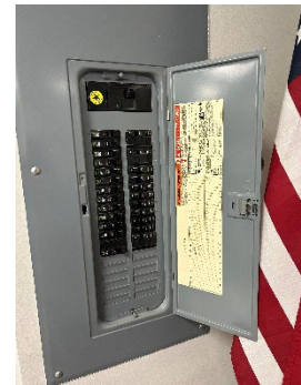
Main Electrical Service
