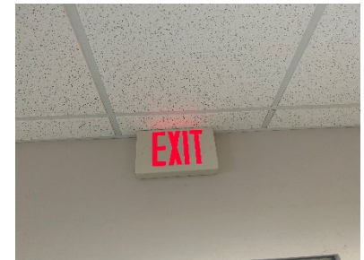
Existing Exit Light
