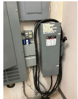
Mobile Generator Connection
