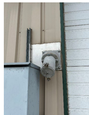
Mobile Generator Connection
