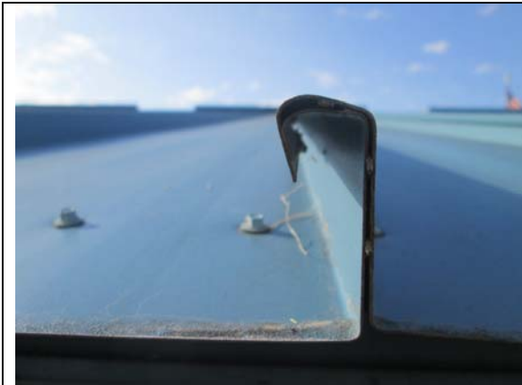
3. Poor seaming of panels
