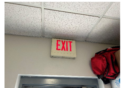
Existing Exit Light
