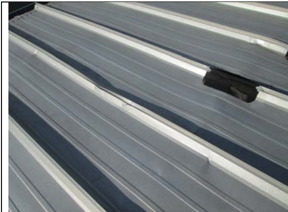
5. Typical panel damage
