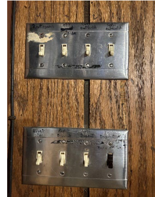
Existing Exterior Lighting Controls
