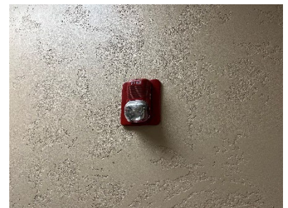
Existing Fire Alarm Horn/Strobe
