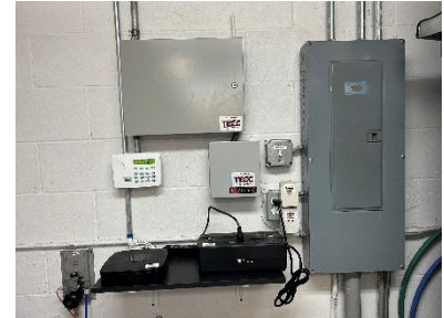
Existing Keyless Entry and Security/CCTV system
