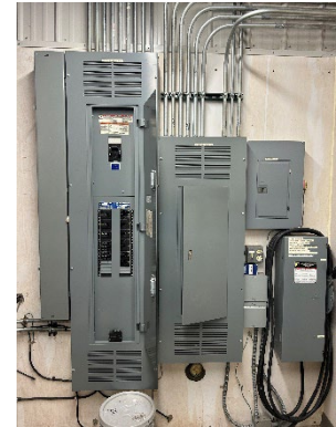
Main Electrical Service
