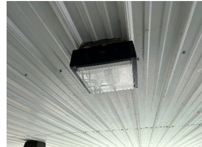
Existing LED Lighting
