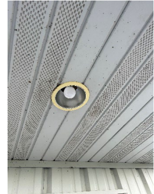
Existing Light Fixture
