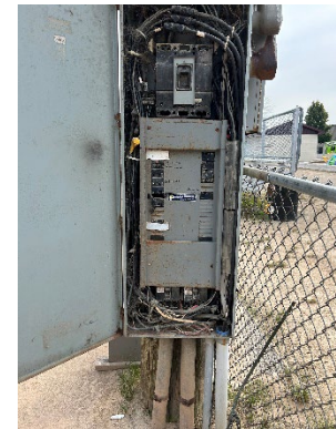
Main Electrical Service
