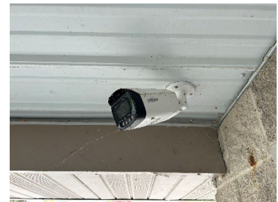
Existing CCTV Camera
