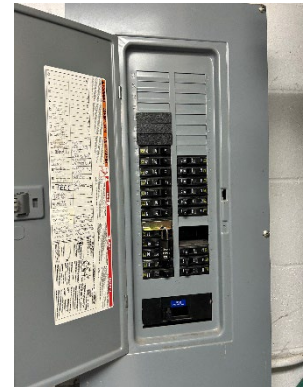
Main Electrical Service
